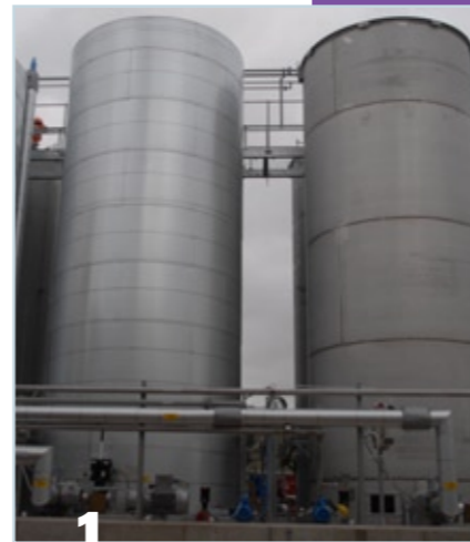
1. Designing in' failsafes, such as automatic pump cut-off to prevent tank over fill, are an effective step to improving safety.
